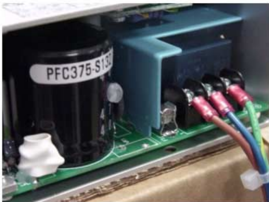
Figure 8. Rear view of the power supply; MOV (VR1) has been removed
